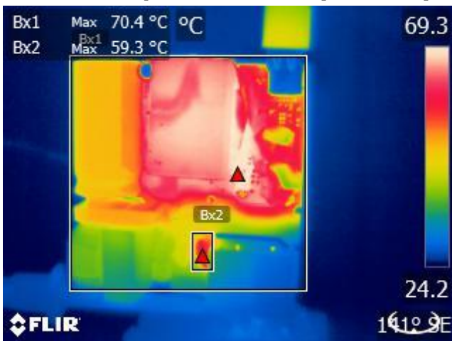
Figure 39 – Top Side Thermal Image. Ambient: 24.6 °C. Bx1: Transformer Winding = 70.4 °C. Bx2: Thermistor RT1 = 59.3 °C.
