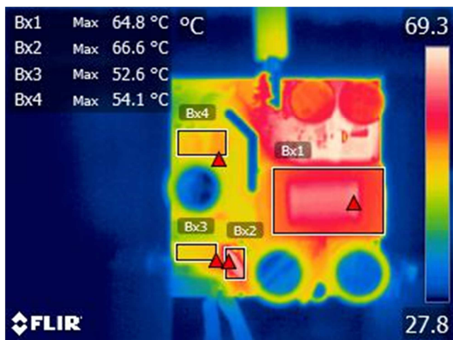
Figure 29 – Top Thermal Image, T_{AMB} = 28.4 °C. Bx1: Transformer, T1 = 64.8 °C. Bx2: Thermistor, RT1 = 66.6 °C. Bx3: CMC 1, L1 = 52.6 °C. Bx4: CMC 2, L2 = 54.1 °C.
